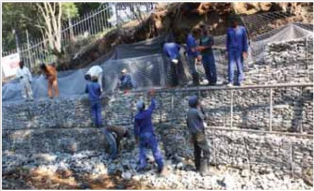
After: Intervention in progress with gabions constructed to support embankment and to prevent further soil erosion.
